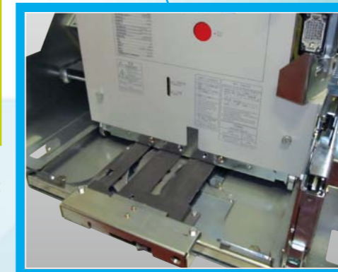
Withdrawable with door closed (Type-M)
